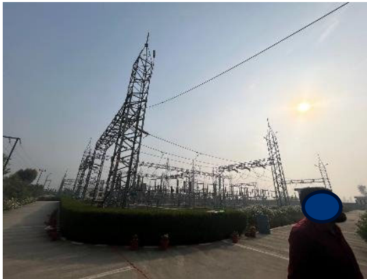
Photo 7: Tilhar Electric Powerstation (Electricity Grid Connection Point)
